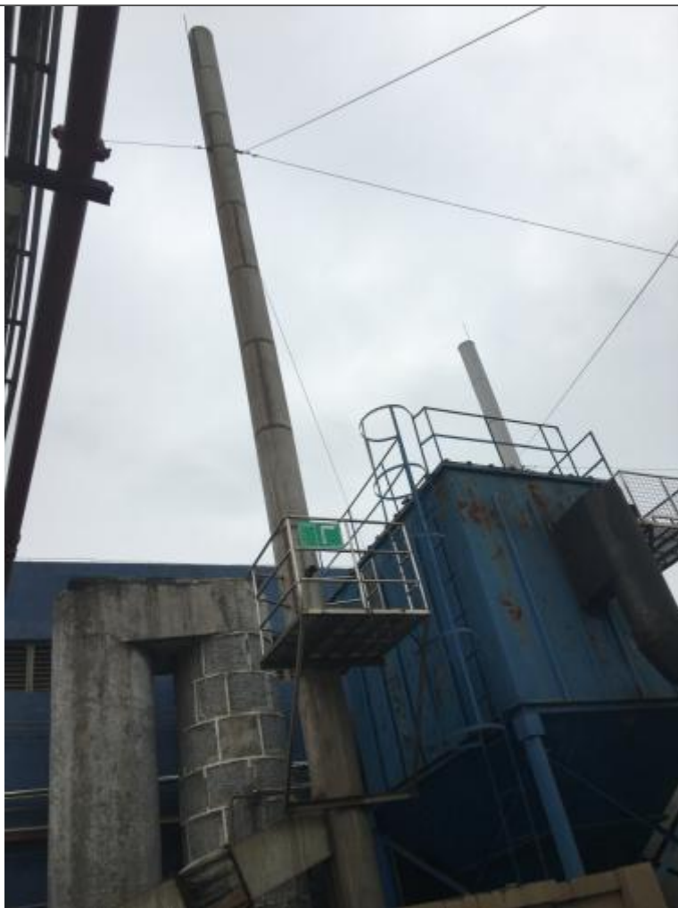
4t/h锅炉烟囱 1#排气筒、布袋除尘+碱液喷淋
