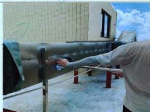
厨房油烟排气筒
