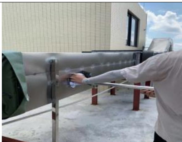
厨房油烟排气筒
